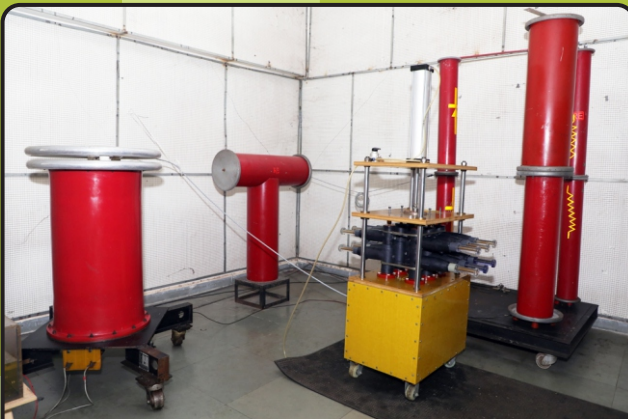
High Voltage Test Lab
